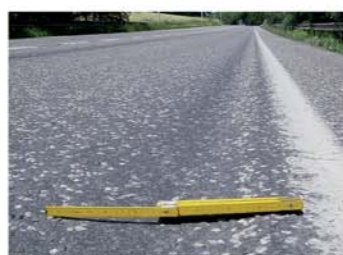
Rutting in an asphalt mixture.
