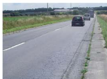
Oxidation in an asphalt mixture.
