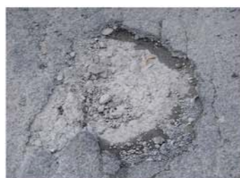
Aggregate stripping as a consequence of moisture induced-damage.
