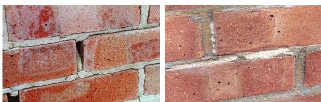
Figure 2. Durability testing after 4 years. On left: mortar without lime. On right: mortar containing lime.
