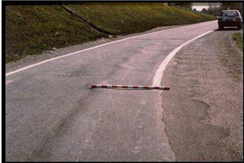
Figure 15: Rutting in an asphalt mixture (from [45]).
